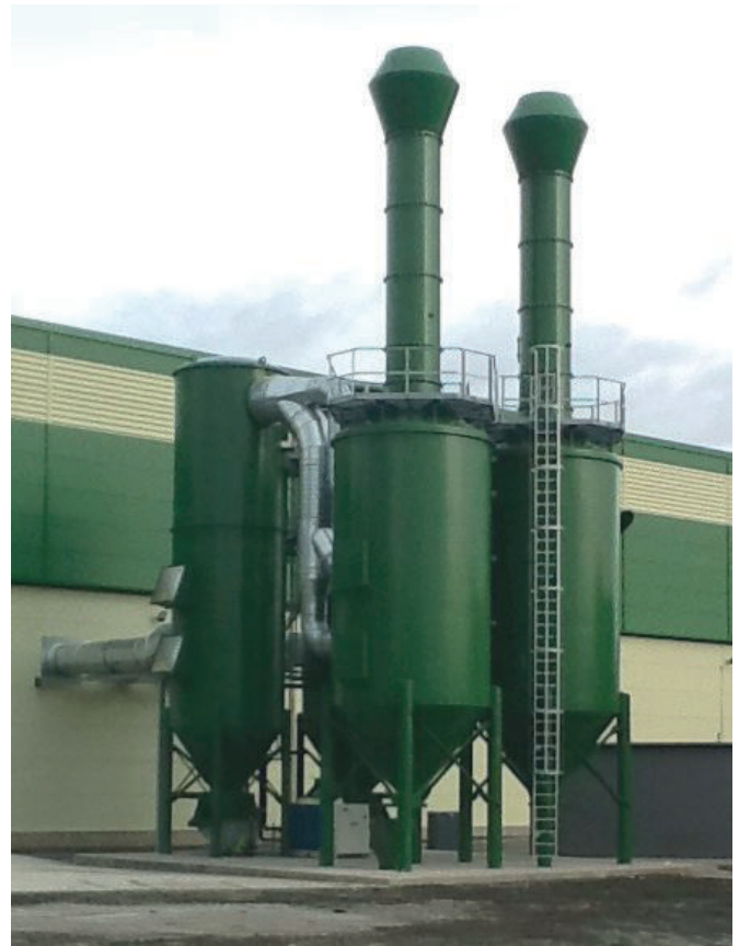
Activated carbon filter 2 x 45,000 m 3 /h
