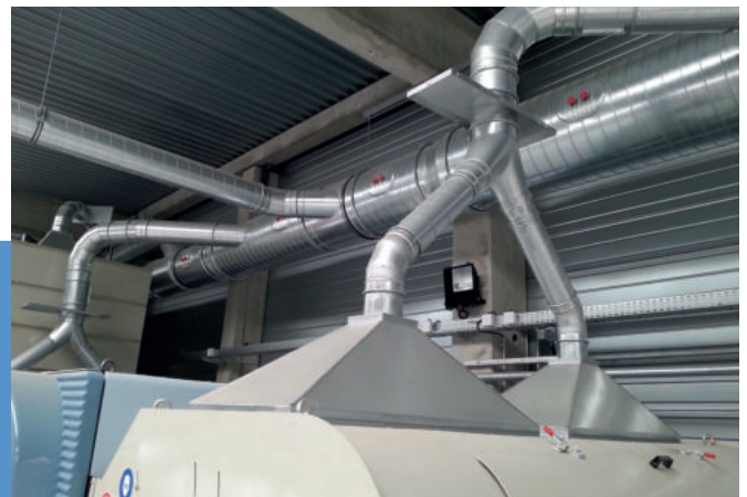
Pipelines and suction hoods
